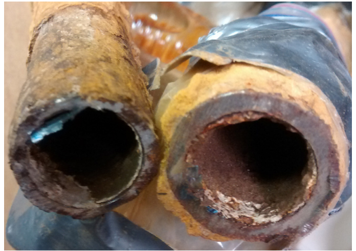
Corrosive water from the Flint River caused aging pipes to leach lead into drinking water, leading to a severe increase in lead poisoning. Photo: Siddhartha Roy/FlintWaterStudy.org.
